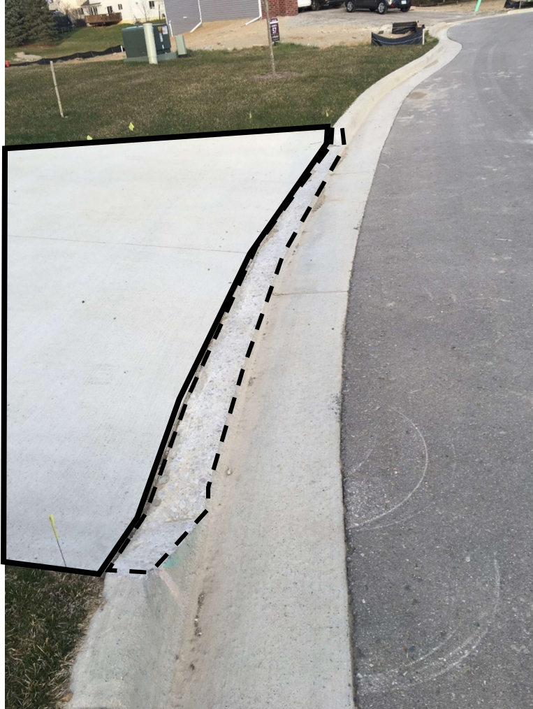
Figure 1 An example of the type of driveway street-end reconstruction to ease vehicle ingress/egress showing cut curb (bounded by a dashed black line) and partially depicted reconstructed bottom section with gradient down to the lower curb (bounded by a solid black line)
